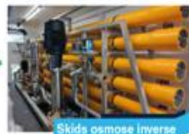
Skids osmose inverse
